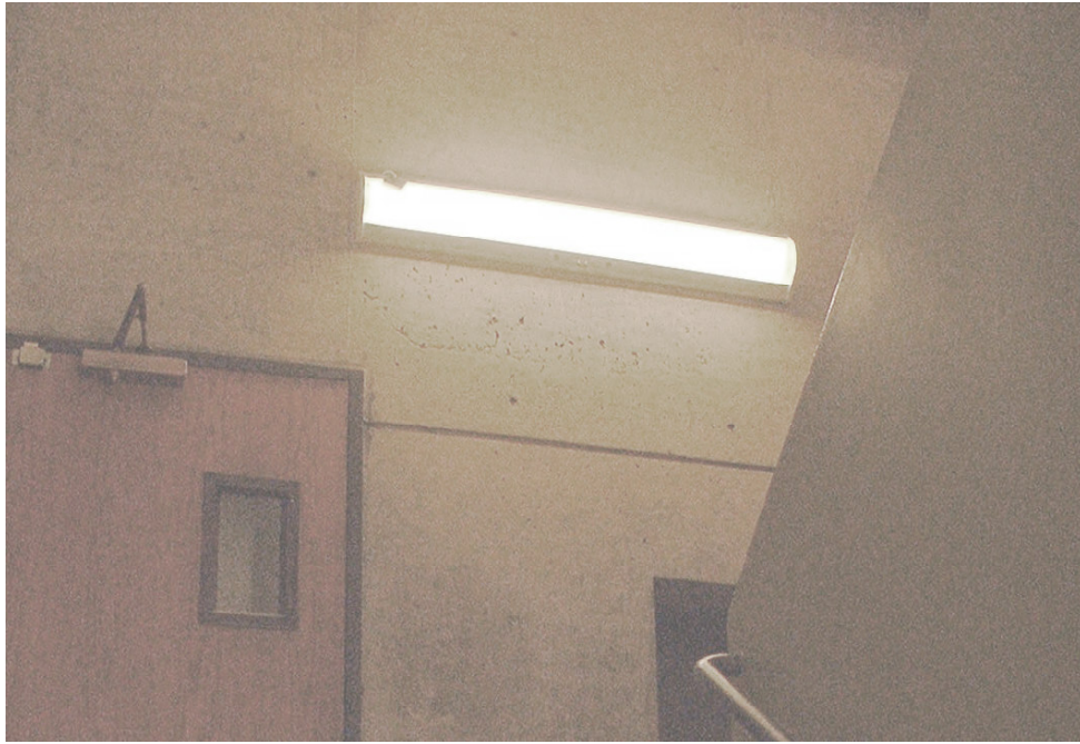
Figure 1. New fixture at Evans 3 rd floor, showing doorway logger and new fixture
