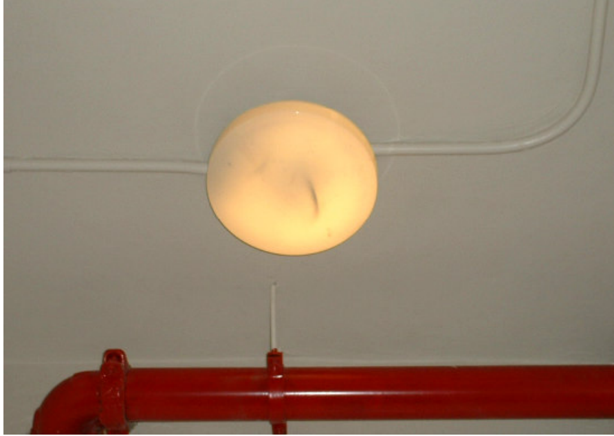
Figure 2. Old fixture at Chiron Building M, first floor
