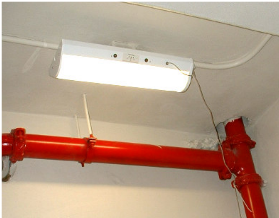
Figure 3. New fixture at Chiron Building M, first floor
