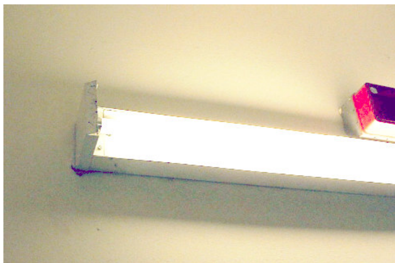
Figure 4. Old fixture at Alameda County GSA building (Lakeside)
